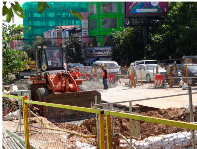
Figure 2. Laying pipes. Intersection of Sihanouk and Monivong Blvds. Photo taken by author.
